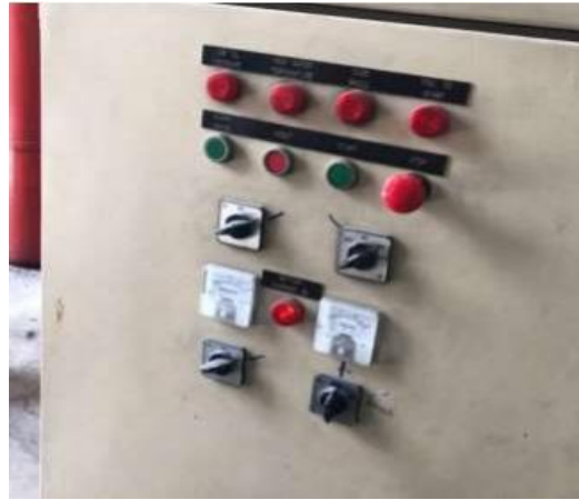
FIG 2 SWITCHES CHARGER PANEL
